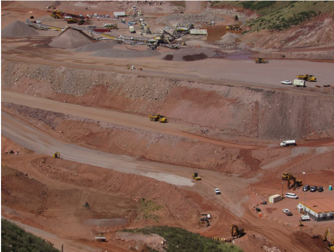
The Chimney Hollow Reservoir under construction in Colorado's Larimer County, July 8, 2022. Credit: Jerd Smith, Fresh Water News
